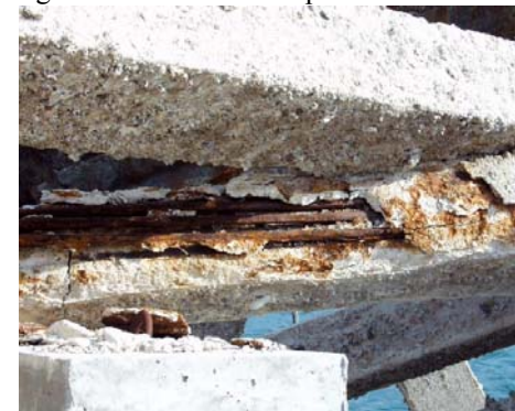
Figure 6. Columns with corrosion damage
